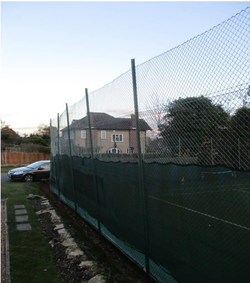
Boundary fence to be replaced
